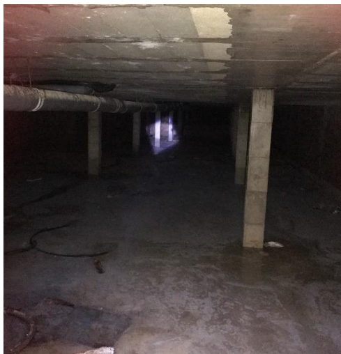
Figure 1: Water under N1.
